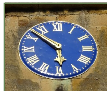
St. James PCC would like to thank all those who contributed to the fund to restore the clock face. Without these donations, the project would not have taken place.
